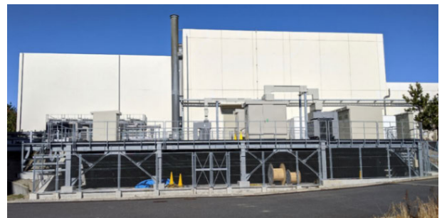
Figure 2. The construction of the new electric sub-station was completed in FY2019.
