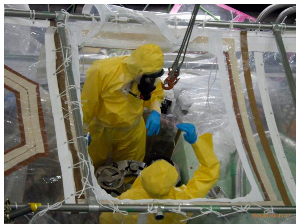
Figure 2. A snapshot of the MUSE target team working on the target replacement assembly, where the radiation workers wearing airtight suites are in a temporary greenhouse to contain radioactive contaminants.
