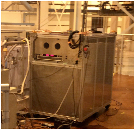
Fig. 1 New 90 kJ Capacitor Bank
