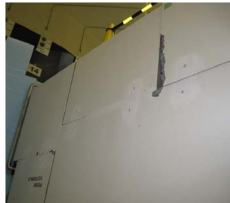
Figure 2. A crack in the shield.
